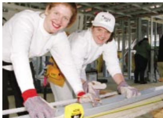
VOLUNTEER TEAMS OF WOMEN WORK TO BUILD AFFORDABLE HOUSING IN WESTERN SYDNEY USING STEEL FRAMING MADE FROM ZINCALUME® STEEL.
